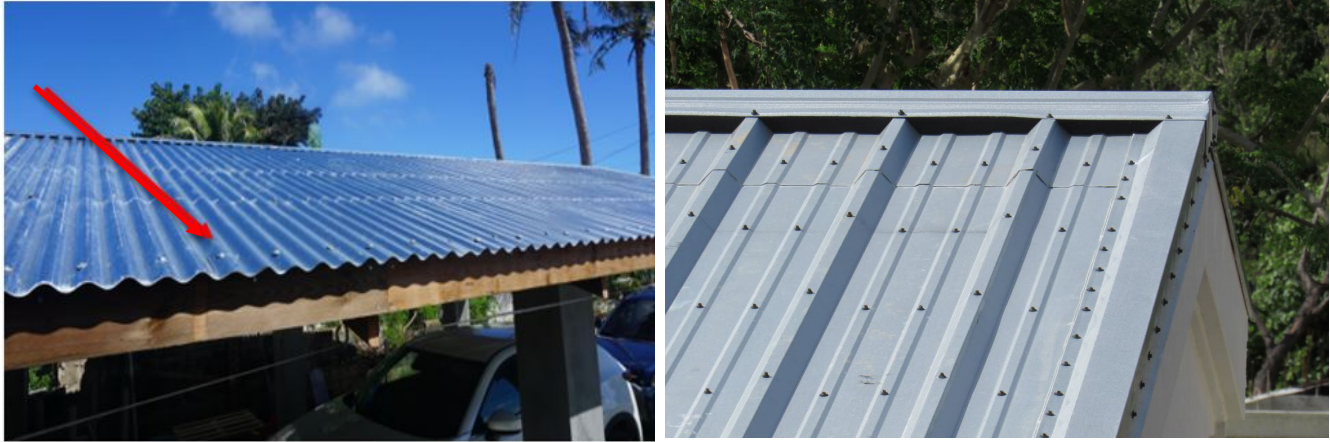
Figure 6: Left—Homeowner construction of corrugated roofing in Koblerville showing better attention to fastener patterns. The perimeter fasteners should have been doubled, but this is a good start. Right—Roof showing good attention to increased fasteners at the edges.
