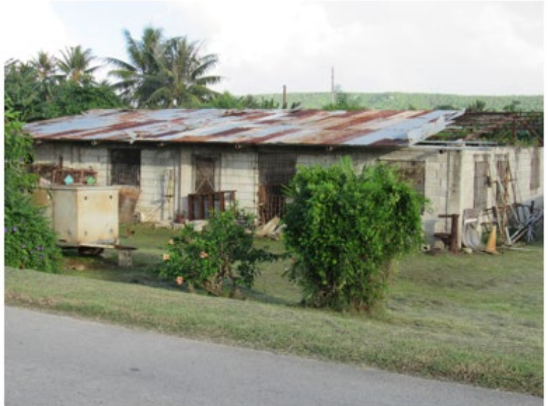
Figure 3: Corrugated metal roofing typical for the CNMI. Note the absence of roof decking or sheathing under the metal roofing as is required for load transfer. This is not good practice.
