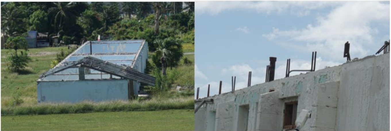
Figure 10: Home on Tinian that used informal roof-to-wall connections. The residential building lost the roof framing during high winds. The roof-to-wall connectors failed to secure the roof framing to the top of the wall.
