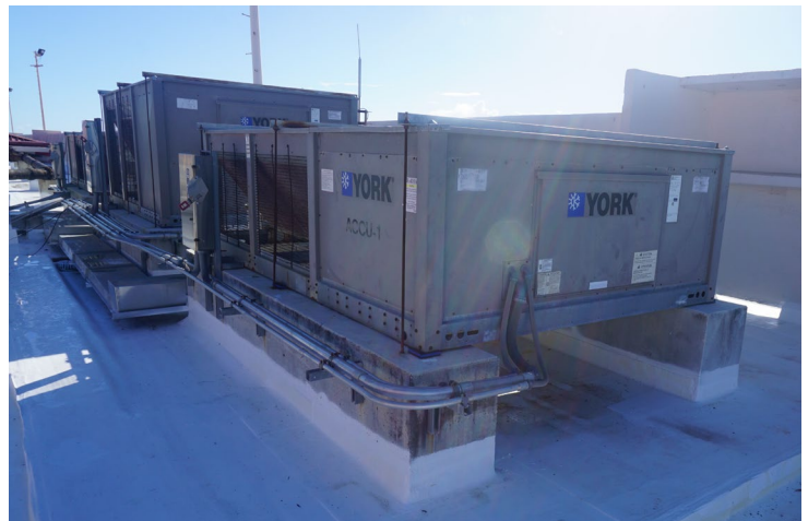
Figure 4. Well-anchored mechanical equipment at Saipan Airport using beams and tie rods.
