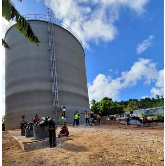
Figure 4.4-6. New 750,000-gallon pre-stressed concrete water tank in San Vicente. Photo by Bryan Manabat as published in the Mariana Variety on Dec 31, 2021 (accessed online).
