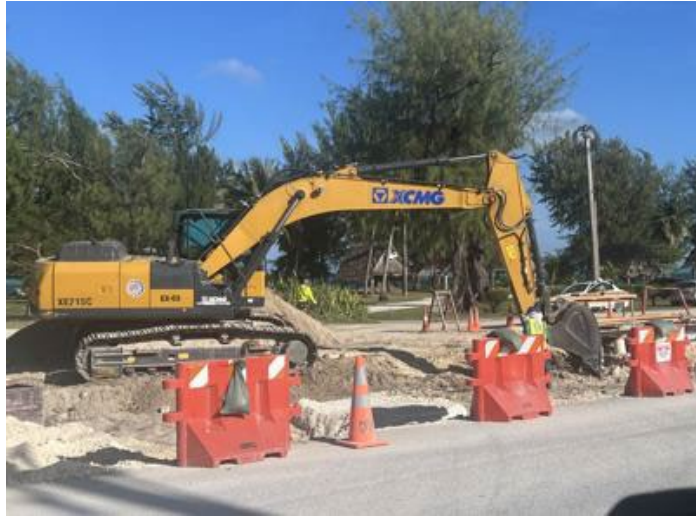
Figure 4.5-17. Mitigation project to improve Beach Road (Route 33), which include repairing existing drainage to enhance flood plain development.
