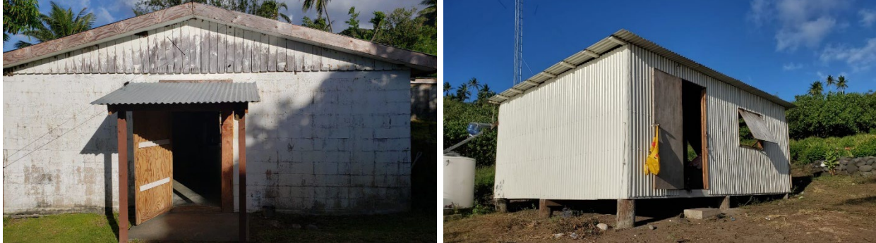
Figure 2.19. Public facilities constructed by the Northern Islands Mayor’s Office on Agrihan (left) and Alamagan (right).
