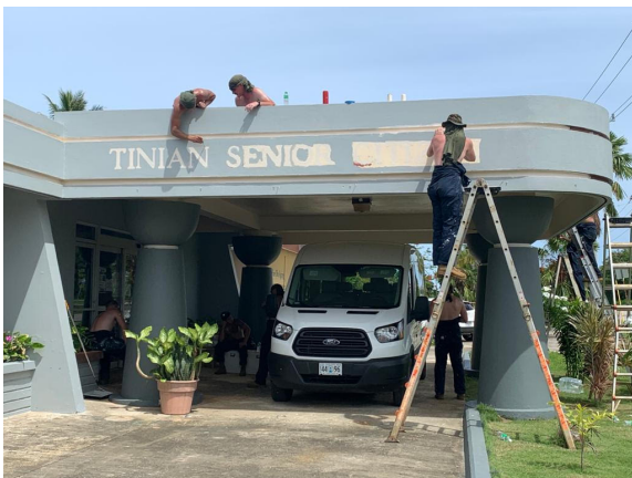
Reopening of the Tinian Senior Center made possible through the Community Relations (COMREL) Partnership with the NMCB Seabees and the Marines 7th Engineer Support Battalion. Renovation included roof repair, painting and replaced kitchen sink to meet FDA/ADA requirements.
