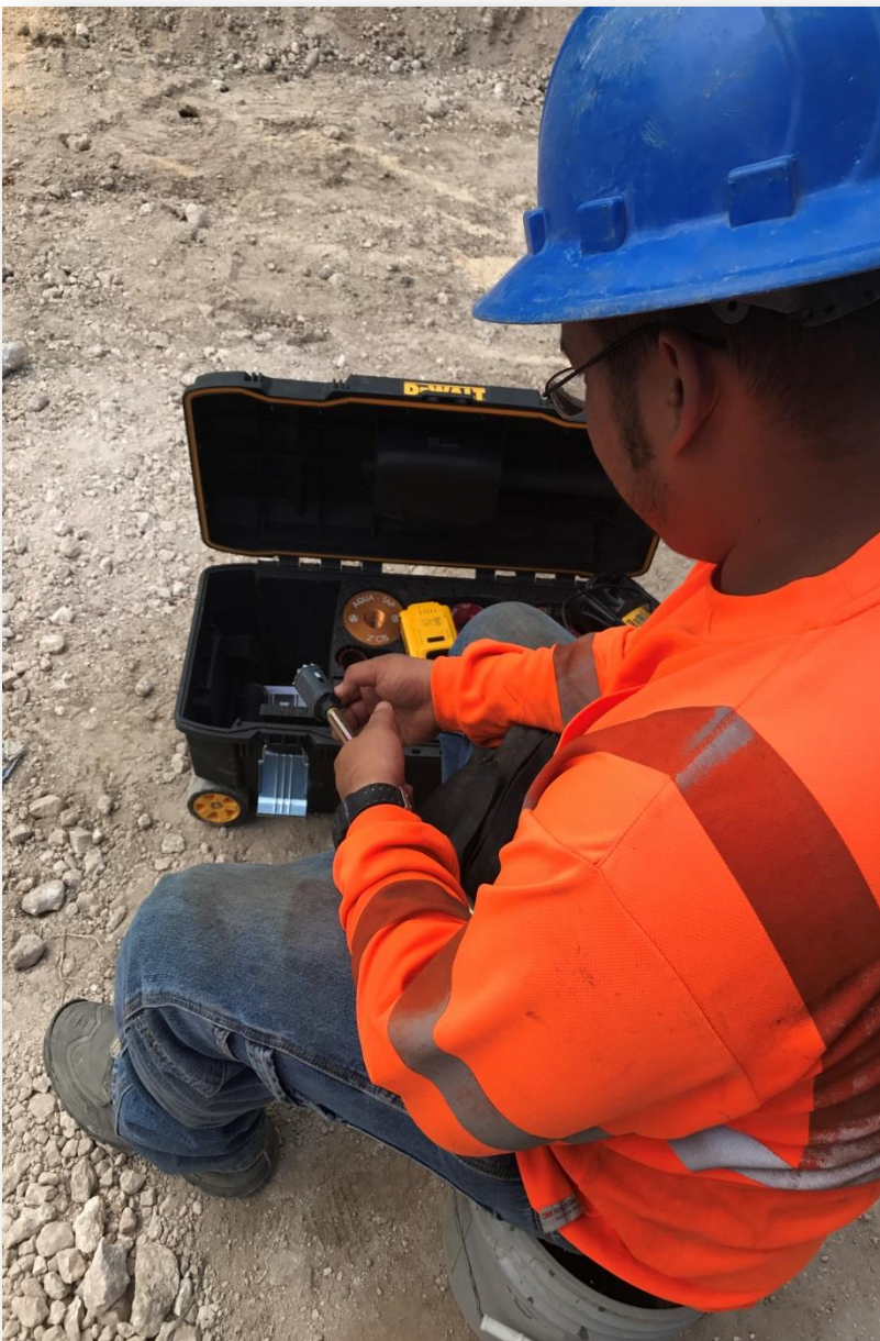
Service Installation Crew Leader Victor Jude (VJ) Concepcion prepares to tap into a main water line to install a water connection to a customer.
