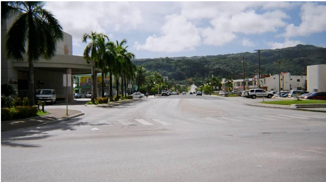
Figure 30: Faded Crosswalk Markings and Poor Pavement Conditions
