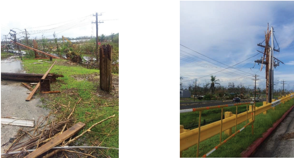
Figure 2. Damaged power poles during Typhoon Yutu along Middle Road / Chalan Pale Arnold (Route 30)
