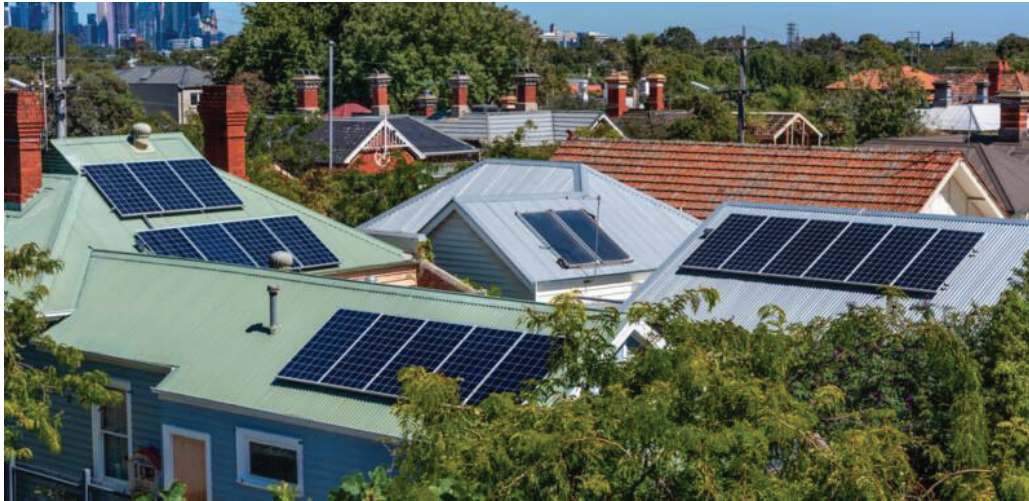
Figure 9. Solar PV Modules Installed on Residential Rooftops
