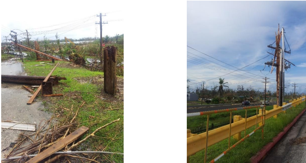
Figure 2. Damaged power poles during Typhoon Yutu along Middle Road / Chalan Pale Arnold (Route 30)
