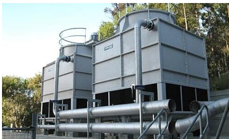
Building cooling equipment
