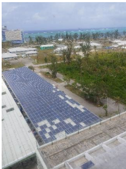
Figure 56. Damage from Typhoon Yutu to the solar PV system at the Marianas Business Plaza.
