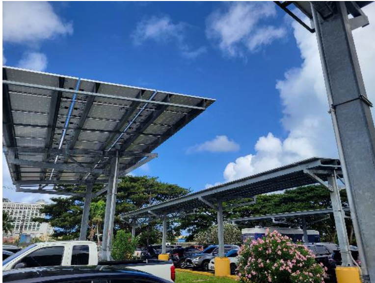
Figure 14. CHCC carport solar PV system.
