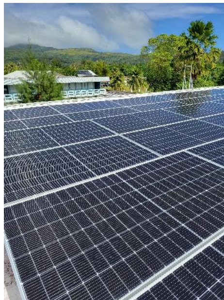
Figure 15. Solar PV panels installed at a Marianas High School building.
