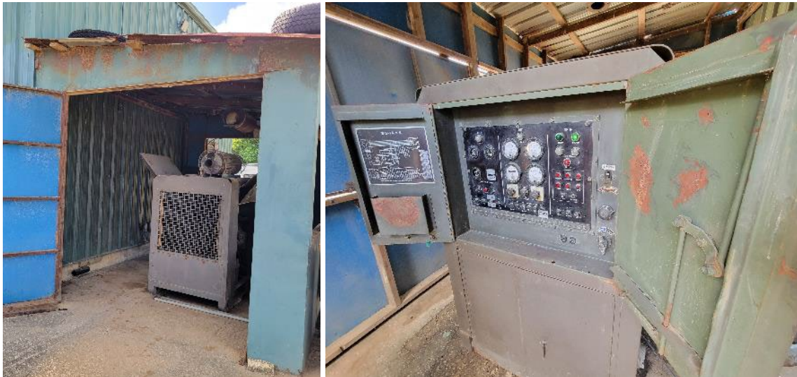
Figure 59. Rental generator in an enclosure with some corrosion.
