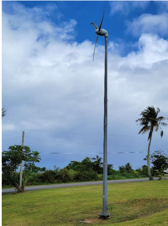
Figure 22. Skystream 2.4 kW wind turbine at the DPW building.
