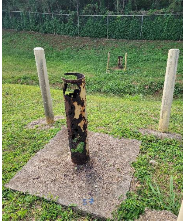
Figure 58. Corroded pipes surrounding water monitoring wells.
