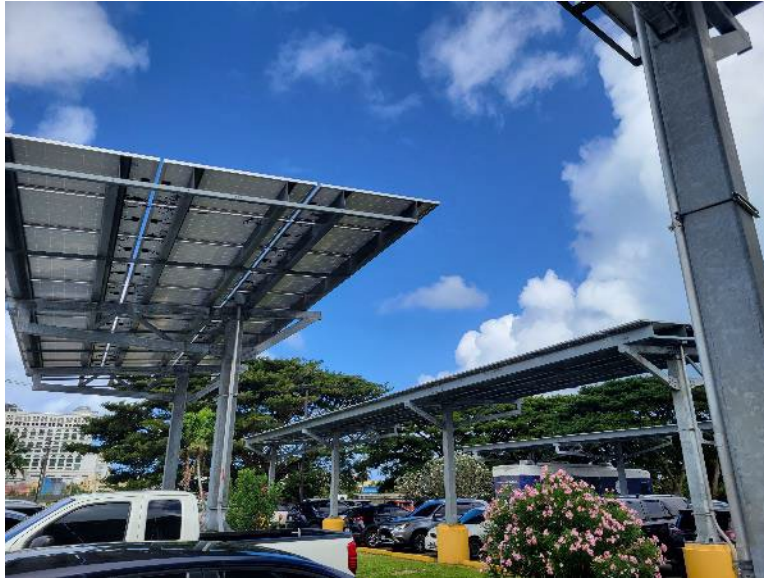
Figure 10. CHCC Carport Solar PV System
