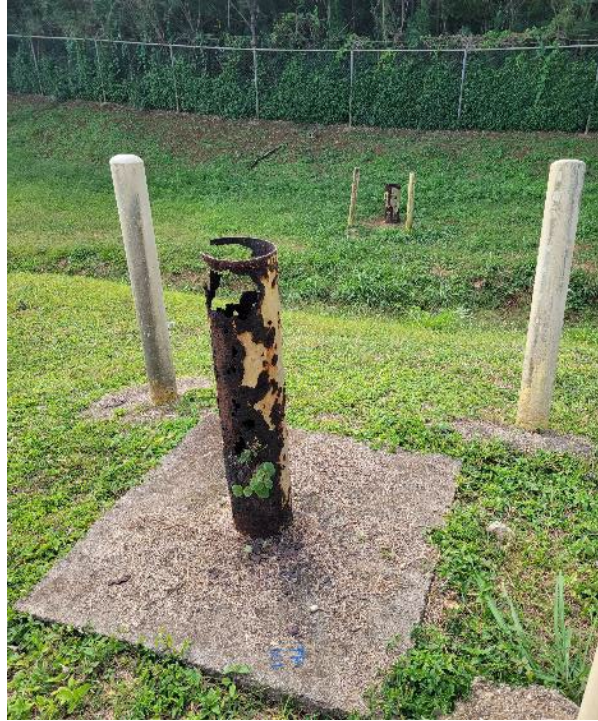
Figure 42. Corroded Pipes Surrounding Water Monitoring Wells
