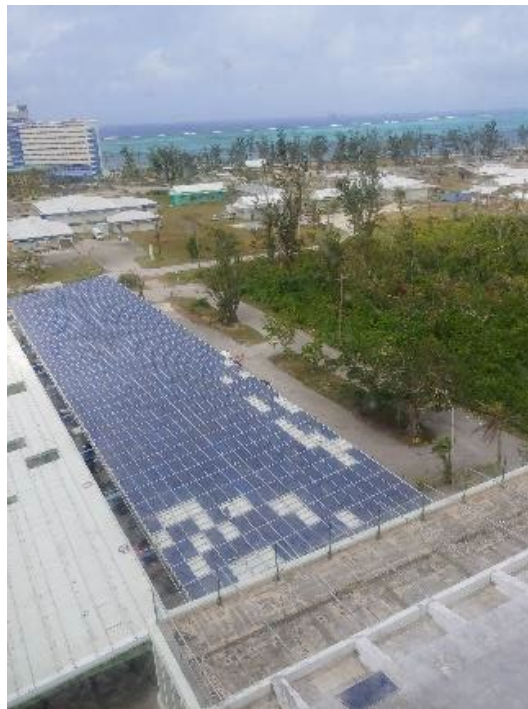
Figure 40. Damage from Typhoon Yutu to the Solar PV System at the Marianas Business Plaza
