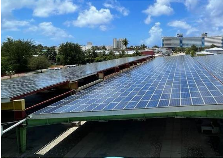
Figure 7. Marianas Business Plaza Solar PV System
