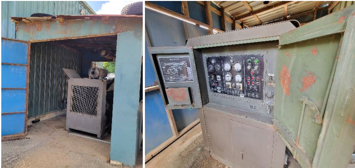
Figure 43. Rental Generator in Enclosure with Some Corrosion
