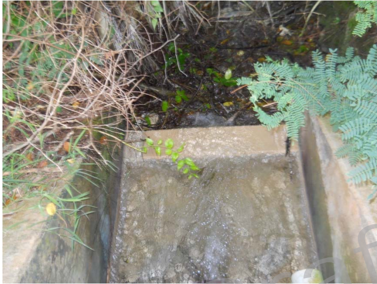
Figure 2.2.3-11. Photo of the Kaan Tank Overflowing during the Wet Season
