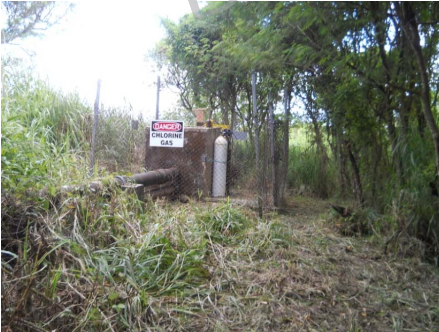
Figure 2.2.2-6. Chlorination System along the Onan Cave Transmission Line
