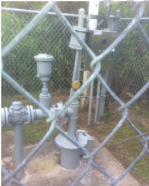
Figure 2.2.2-1. Typical Well Fencing
