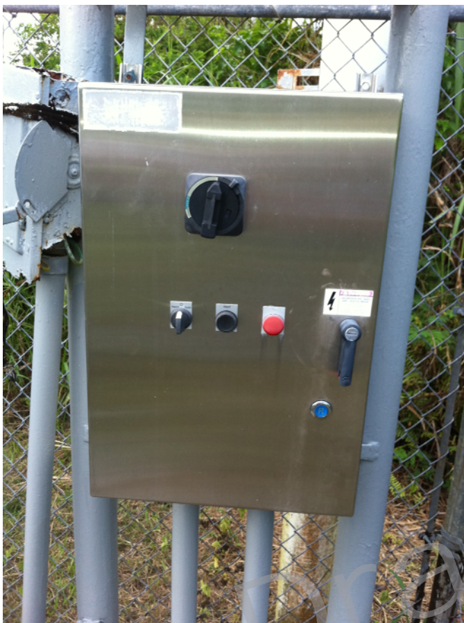
Figure 2.2.2-2. Typical Well Control Panel
