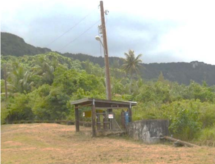
Figure 2.2.2-5. Chlorination System at the Kaan Tank
