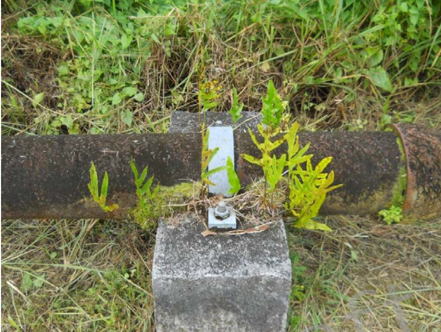
Figure 2.2.2-9. Kaan Transmission Line and Concrete Pedestal
