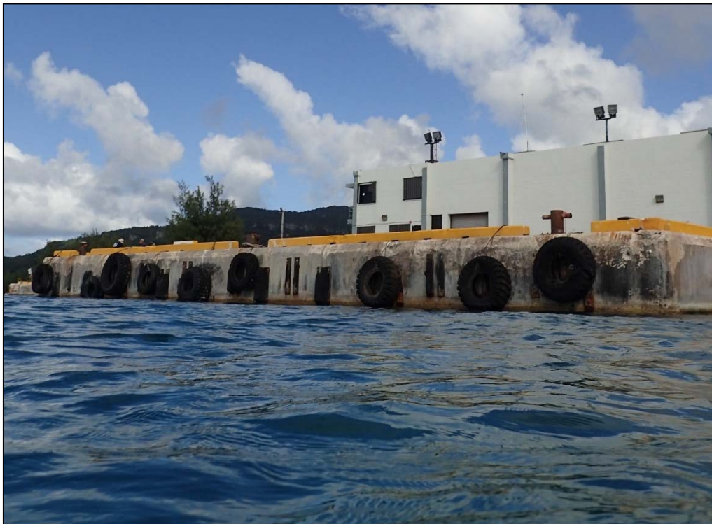
Photo 35. View of the V-fender remnants and added tires suspended from the curbs and cap at Berth 2.
