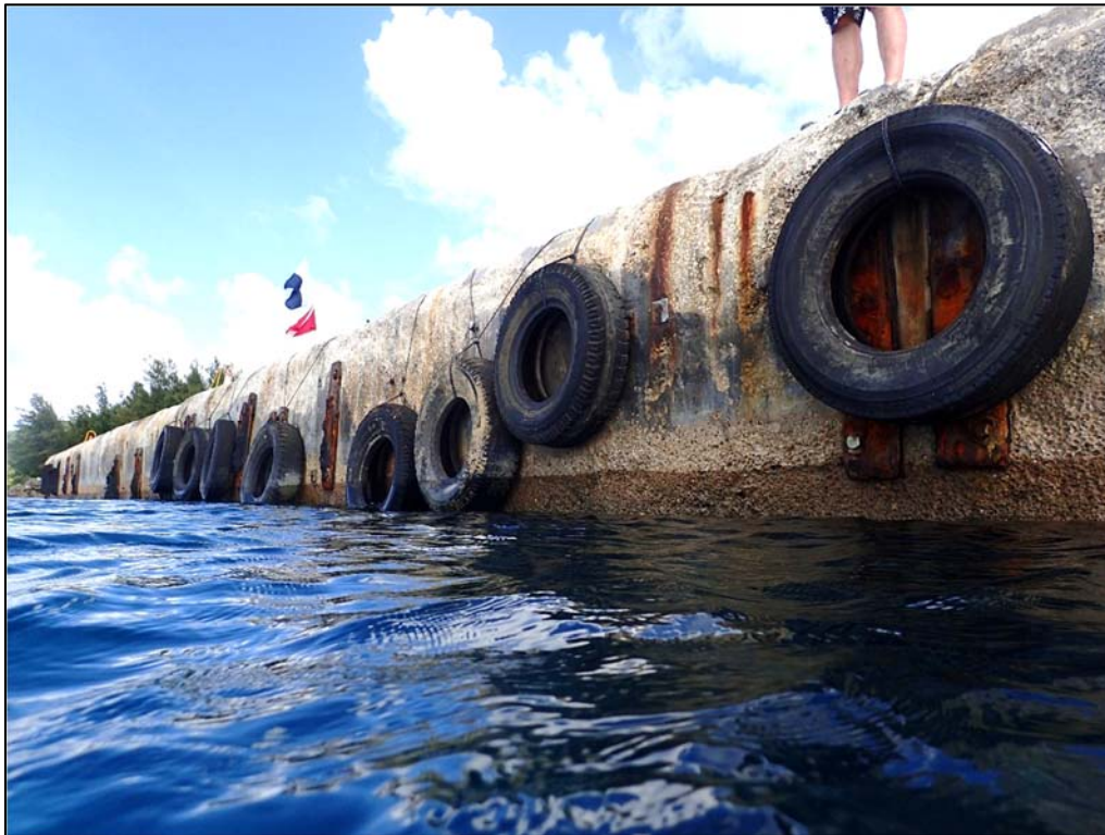
Photo 33. Berth 1. Remnants of failed V-fenders and tires found on the face of Berth 1.
