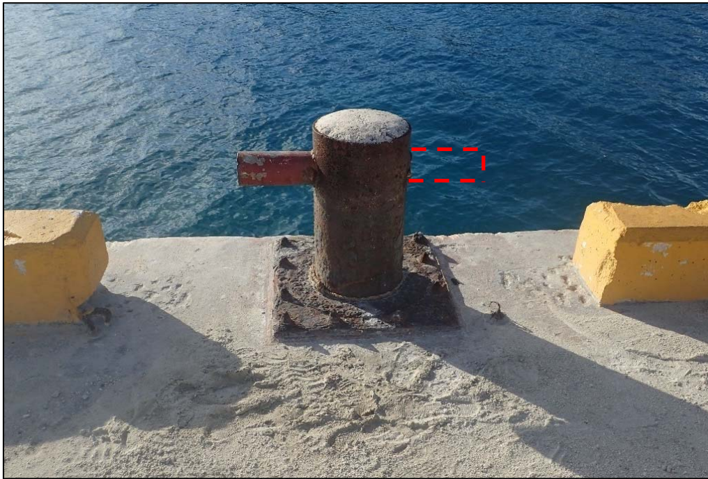
Photo 24. The bollard at Berth 2 Sta. 0+90 is missing a horn (red dashed line). The mooring bollard should be replaced.
