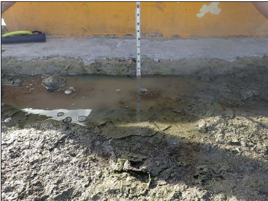
Photo 28. Berth 2. Soil and water collects behind the cap at an area of deck subsidence. The resultant depression is 3-in. deep at Sta. 0+58 and up to 5-in. deep in other areas.
