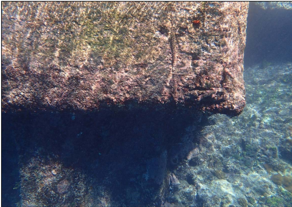
Photo 13. Berth 2 concrete cap. Erosion damage coupled with insufficient concrete cover over the reinforcing steel found at Station 0+00 seen from below water. This damage is typical of north and south corners on each berth.
