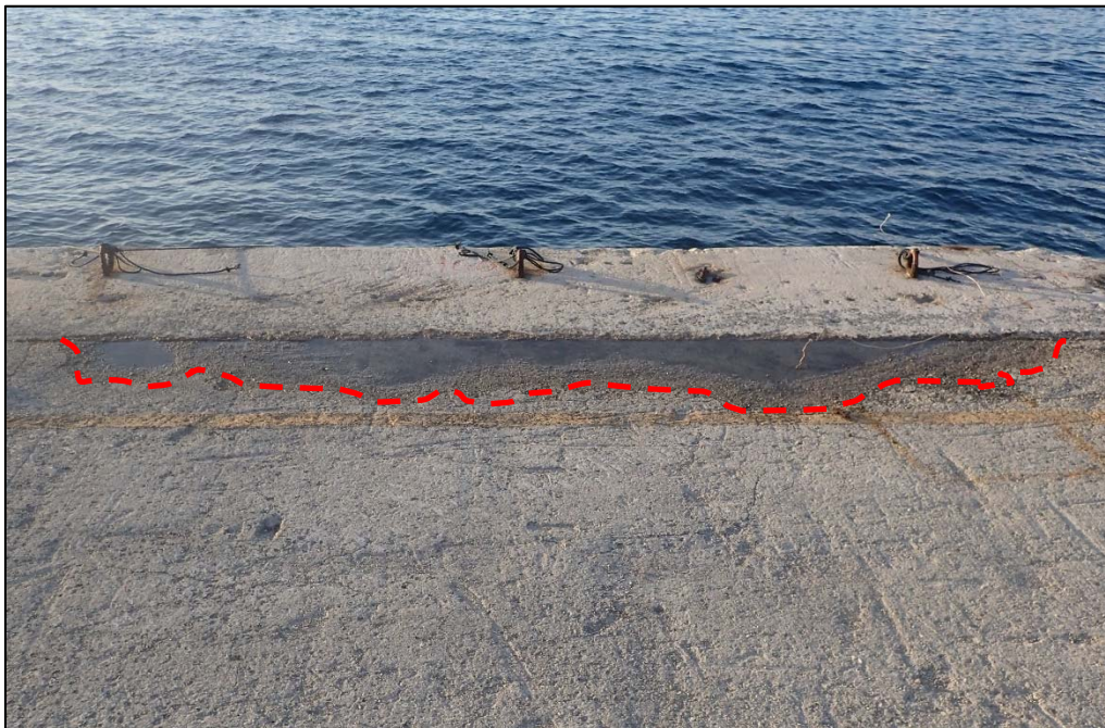
Photo 26. Ponding from deck surface subsidence noted at Berth 1 Station 0+60.
