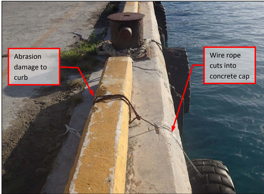
Photo 38. Berth 2 Station 0+55. Wire rope is used to fasten the tire to the curb resulting in abrasion damage to the curb and the corner of the concrete pile cap.
