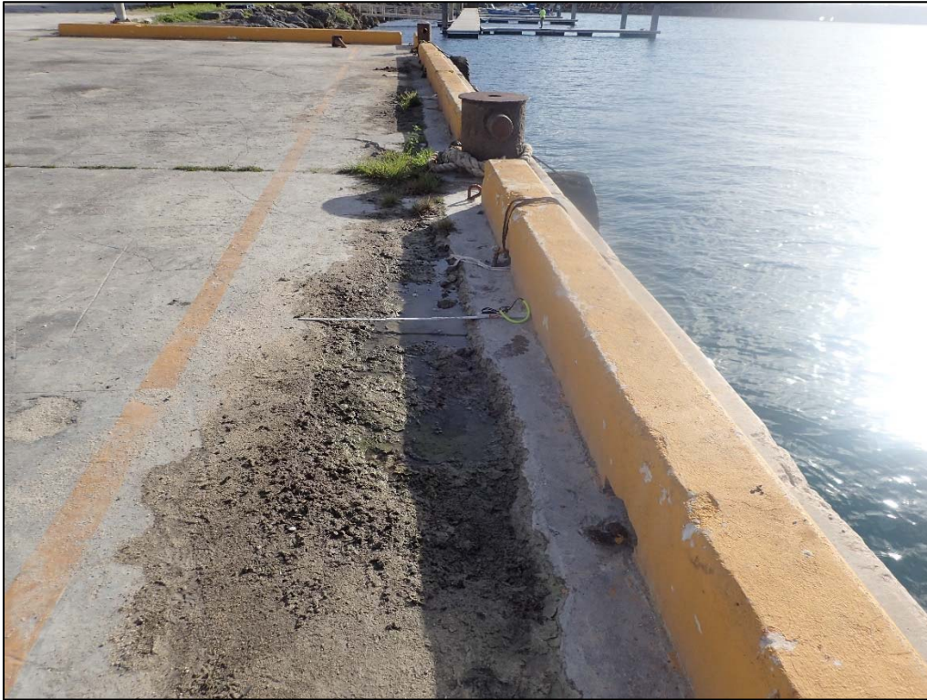
Photo 27. Subsidence behind the concrete cap at Berth 2 looking south.
