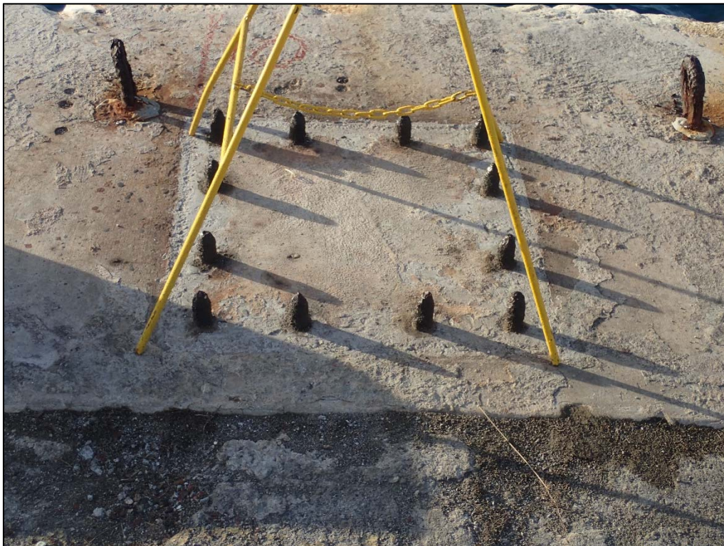
Photo 21. Berth 1 Station 0+10 where a bollard has been removed and the anchor bolts remain.
