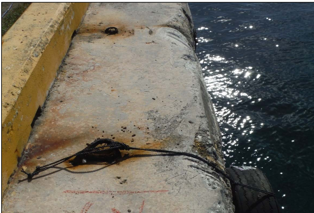
Photo 18. Berth 1 concrete cap Station 0+30 looking south. Typical abrasion damage seen from above deck from wires and chains used to hang tires for makeshift fenders. This is typical of both berths.
