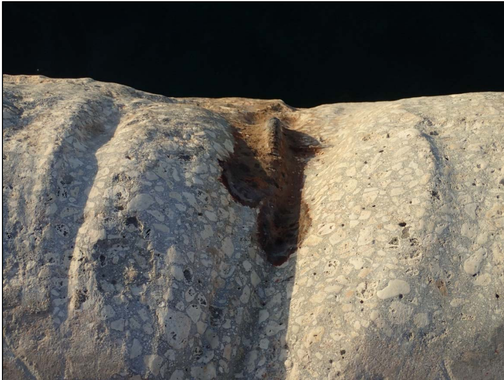
Photo 39. Berth 1 Sta. 1+05. Abrasion damage from hanging tire fenders resulting in exposed reinforcing steel in the concrete cap.
