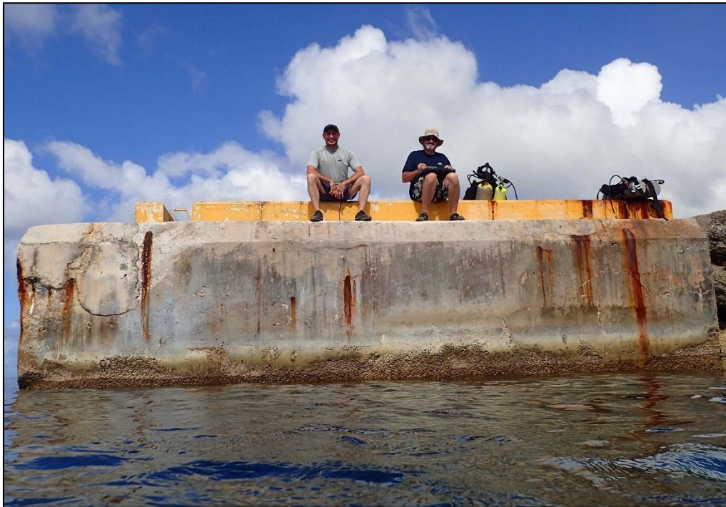
Photo 15. Berth 1 concrete cap. Corrosion spalling and bleeding noted throughout the south face. See Attachment B for further discussion of concrete deterioration.
