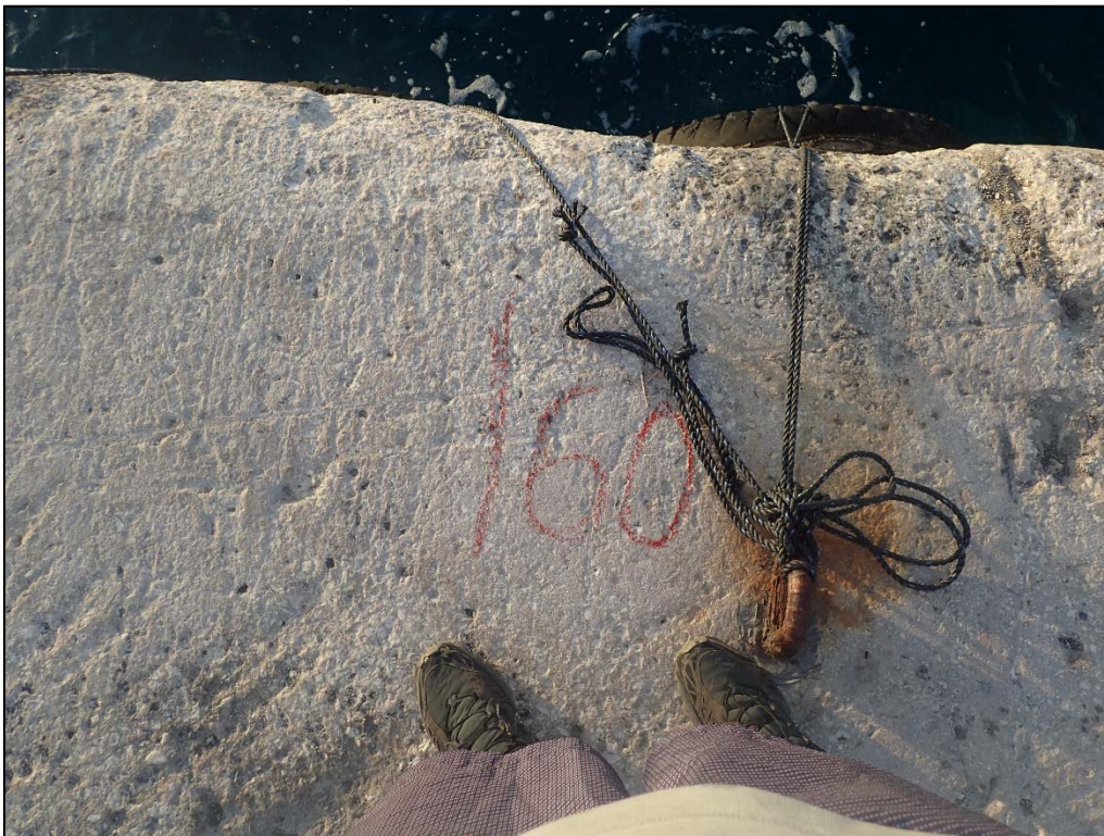
Photo 37. Berth 1 Sta. 0+60. Tires are tied to a pad eye with a polypropylene line.
