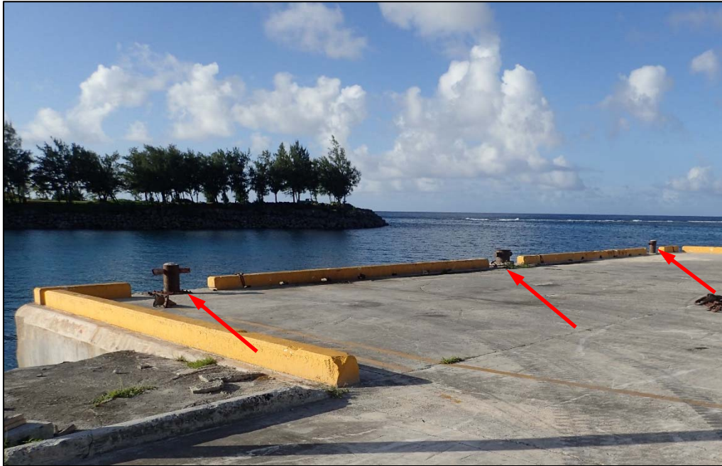
Photo 20. Layout of mooring bollards at Berth 2. Red arrows point to the single bollards at the face of the berth.
