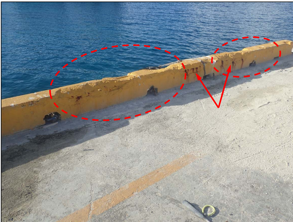
Photo 31. Berth 2. Typical corner spalls (oval) and rust bleeding (arrows) from Sta. 0+64 to 0+80.
