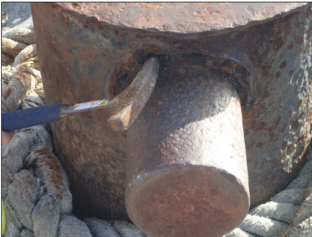
Photo 23. Berth 2, Sta. 0+50. Severe corrosion noted at the weld of the horn to the bollard cylinder. The hammer penetrates an area where there is 100% section loss of the weld material. The mooring bollard should be replaced.
