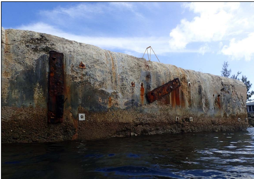
Photo 16. Berth 1 concrete cap. Widespread abrasion damage due to friction on the top of the cap and erosion damage resulting in cement particle/aggregate loss on the lower portion of the cap.
