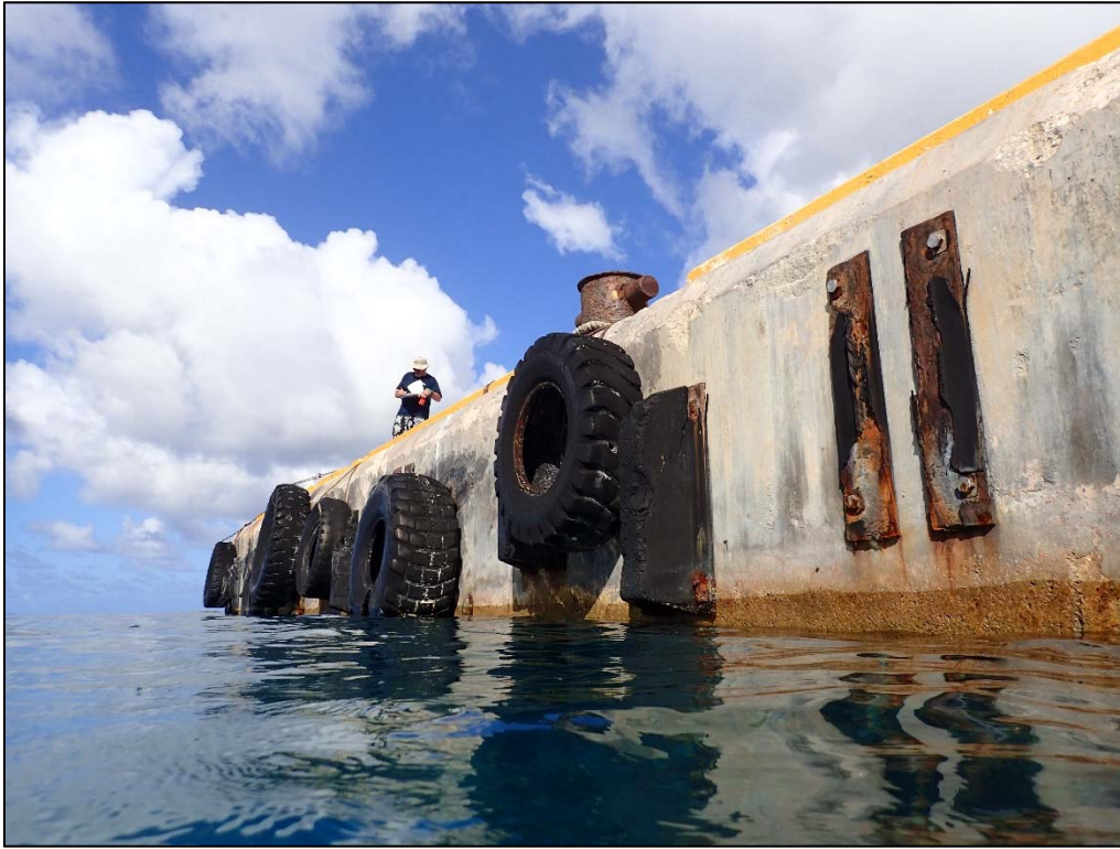
Photo 36. Close up of the V-type fender remnants and suspended tires at Berth 2.
