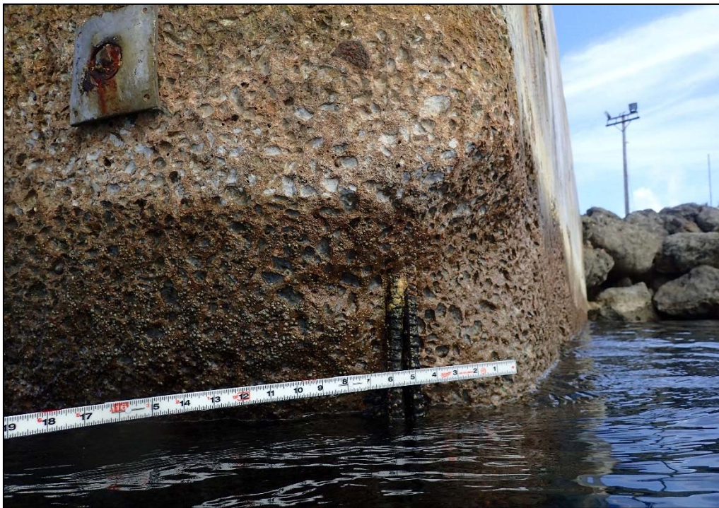
Photo 14. Berth 1 concrete cap. Typical erosion damage where the aggregate has “raveled” away over time leaving rock pockets, found at the southwest corner above the damage seen in Photo 11. This damage is typical of north and south corners on each berth.
