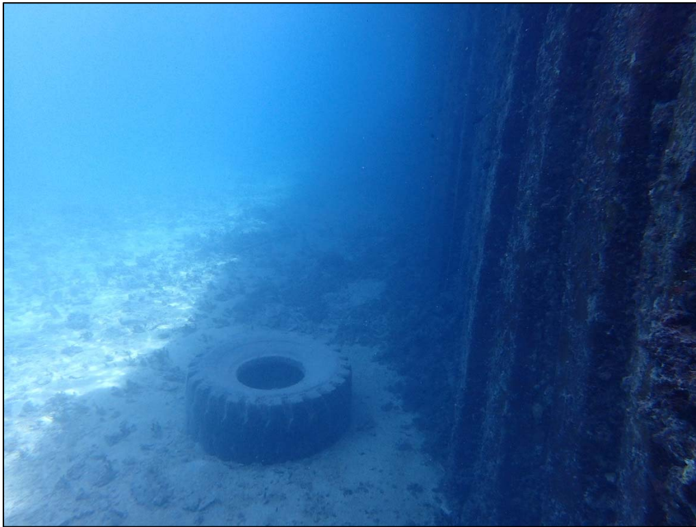
Photo 42. The bottom condition and a tire at Berth 2 Station 0+40.
