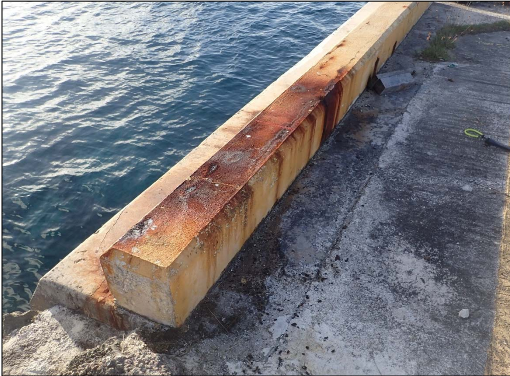
Photo 30. Berth 1. An example of closed corrosion spalling indicated by the orange staining and cracks at the edges of the curb on the south side.
