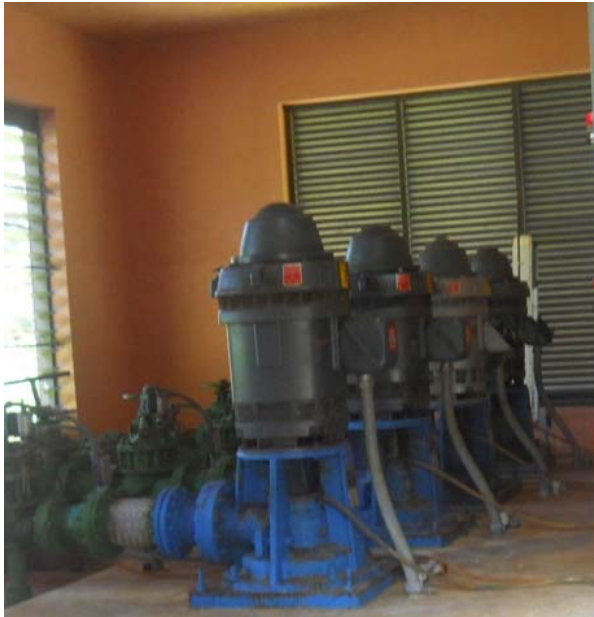
Figure 2.2.2-2. Maui II Booster Pumps
