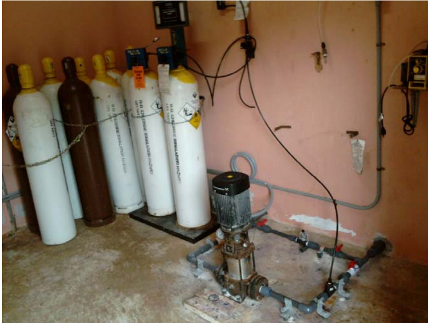
Figure 2.2.2-1. New Maui II Chlorine Injection Pump
