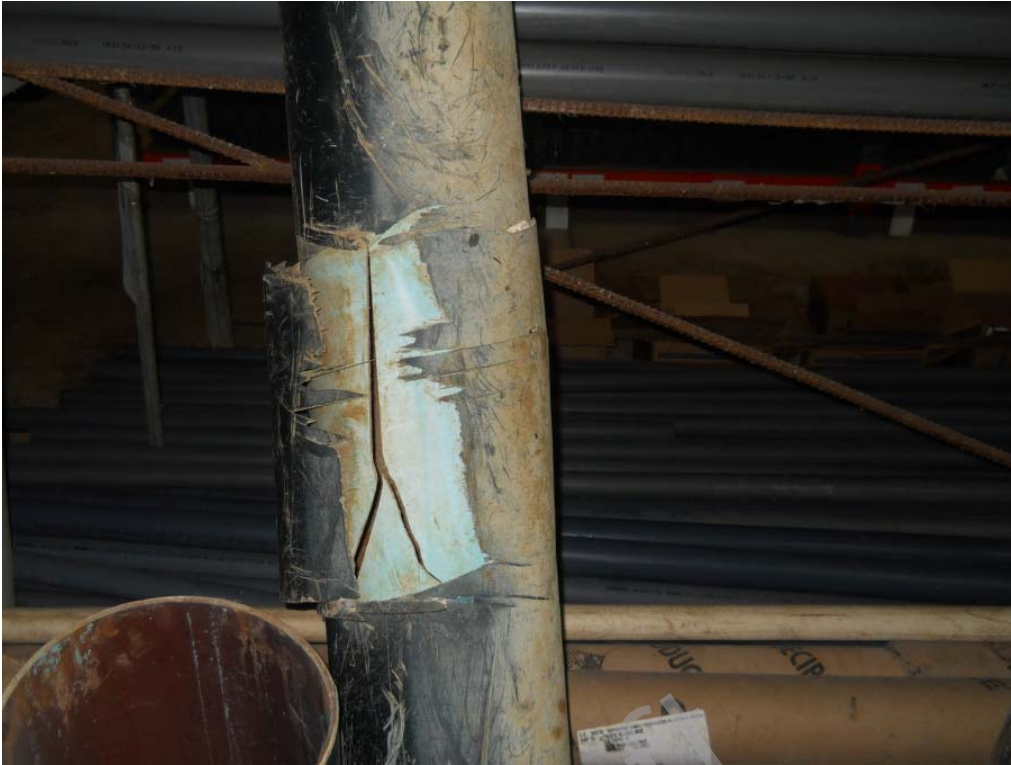
Figure 2.2.2-5. Photo of Longitudinal Cracking between Maui II Pump Station and the HMT
