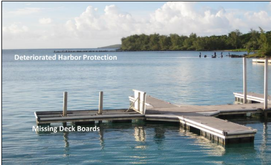
Figure 2-22: Tinian Small Boat Marina Damage
