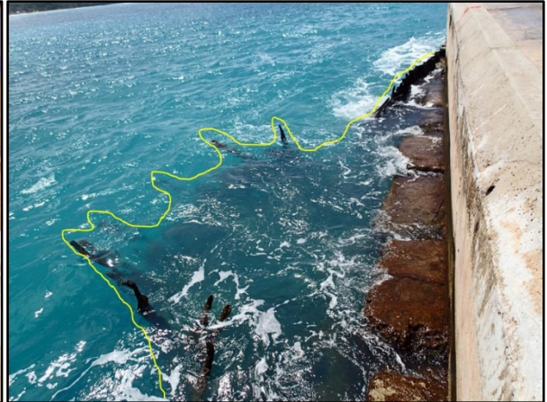
Photo 3-5. North Quay, Berth 4, east-facing wall with failed SSP wall (yellow outline traces the top of the failed SSP wall)
