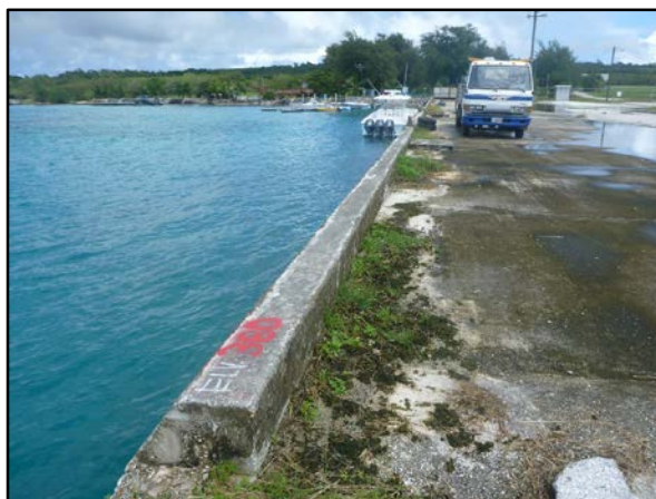
Photo 3-6. North portion of the West Connecting Pier, looking north. This wall is actively used for small boat mooring.
