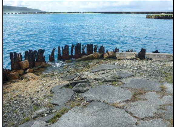
Photo 3-11. Center Finger, southeast corner showing typical conditions of Finger Pier SSP wall.
