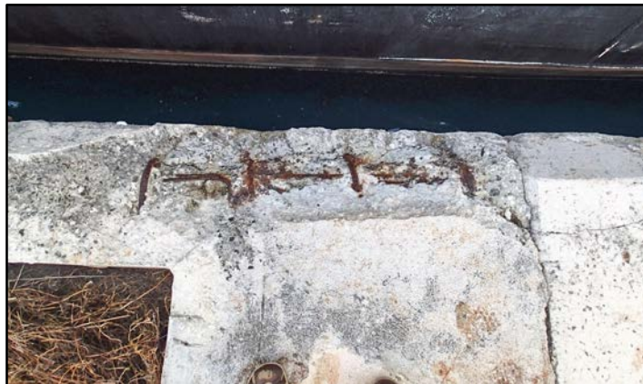
Photo 3-3. North Quay, pile cap/curb. Example of an open concrete corrosion spall.
