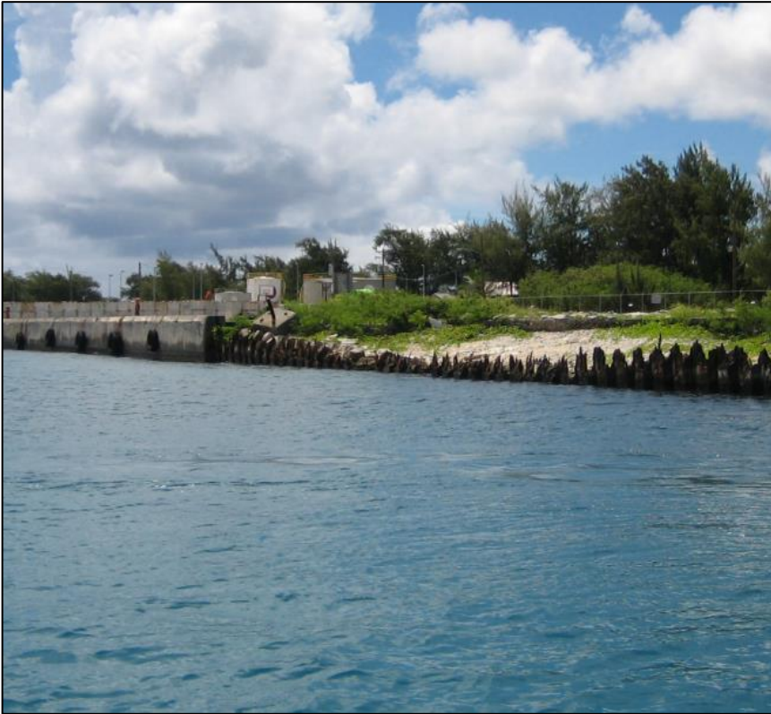
Figure 2-13: Berth 3 Prior to Repair (2006)
