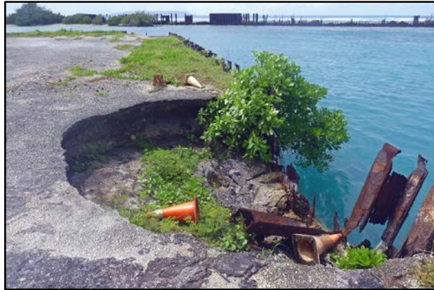
Photo 3-9. Connecting Pier, southwest side, looking south with the breakwater in the background.
