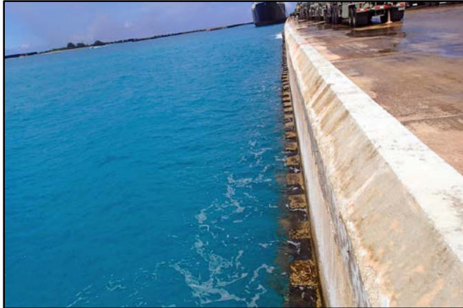
Photo 3-4. North Quay, Berth 4 with SSP wall extends beyond the concrete curb structure.
