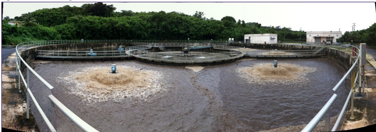
Figure 2.2.3-2. Sadog Tasi WWTP Aeration Basins and Clarifier
