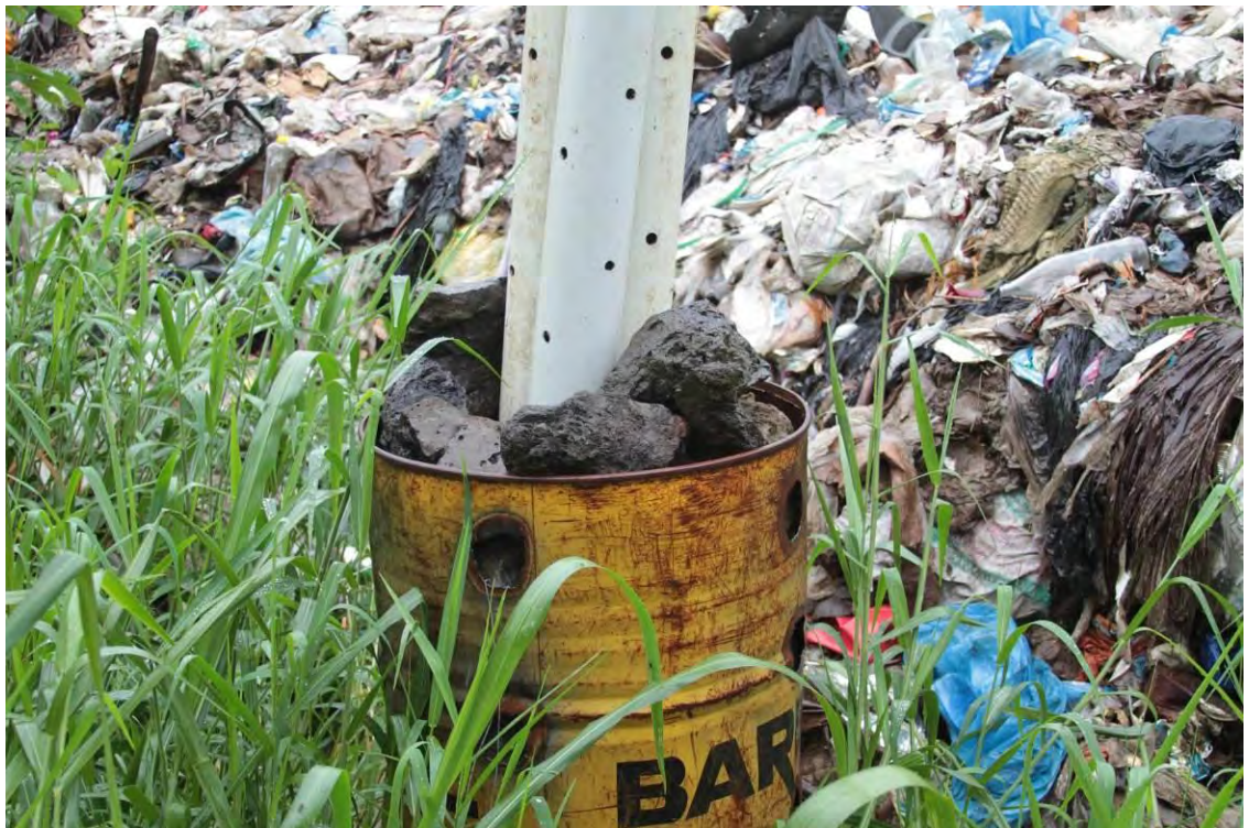
Figure 19. Vertical air/gas vent at the Tafaigata Fukuoka-style Landfill
