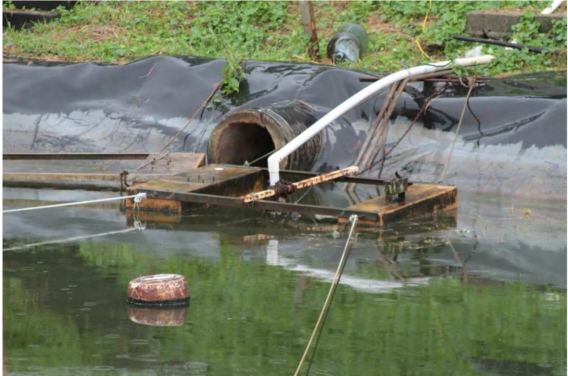
Figure 18. Lined leachate pond at the Tafaigata Fukuoka-style Landfill showing a large-diameter leachate pipe entering from the landfill
