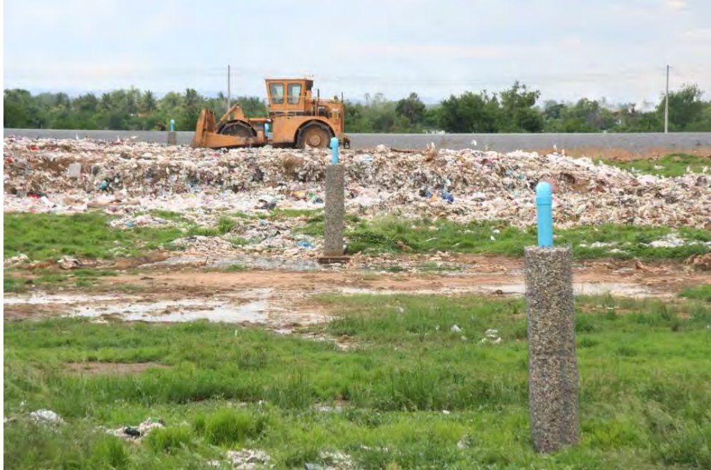
Figure 30. Landfill gas well built with rock encased in wire
