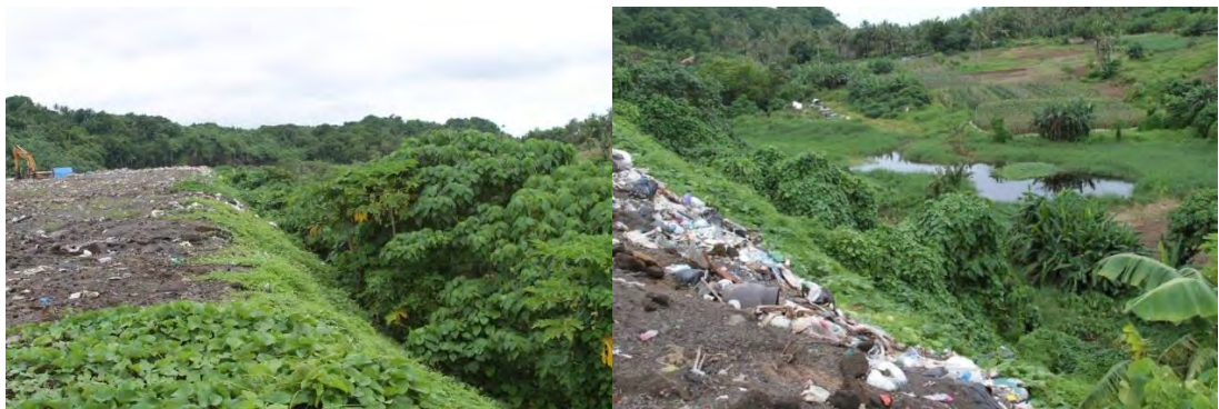
Figure 13. Steep side slopes (left) and leachate ponding (right) observed at the Futiga solid waste facility
