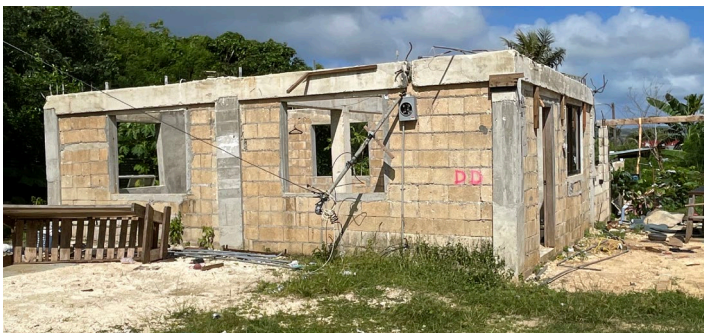
Figure 1. Wind and windborne debris damage to building envelope observed after Super Typhoon Yutu, which hit in October 2018.
